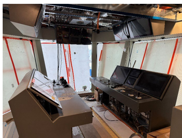
DP console on starboard side
