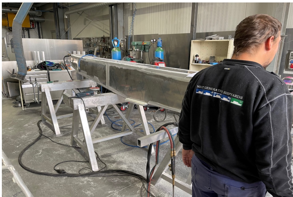
State of affairs in late August. Top: the deck begins to take shape. Bottom: the initial form of the A-frame ©FH
