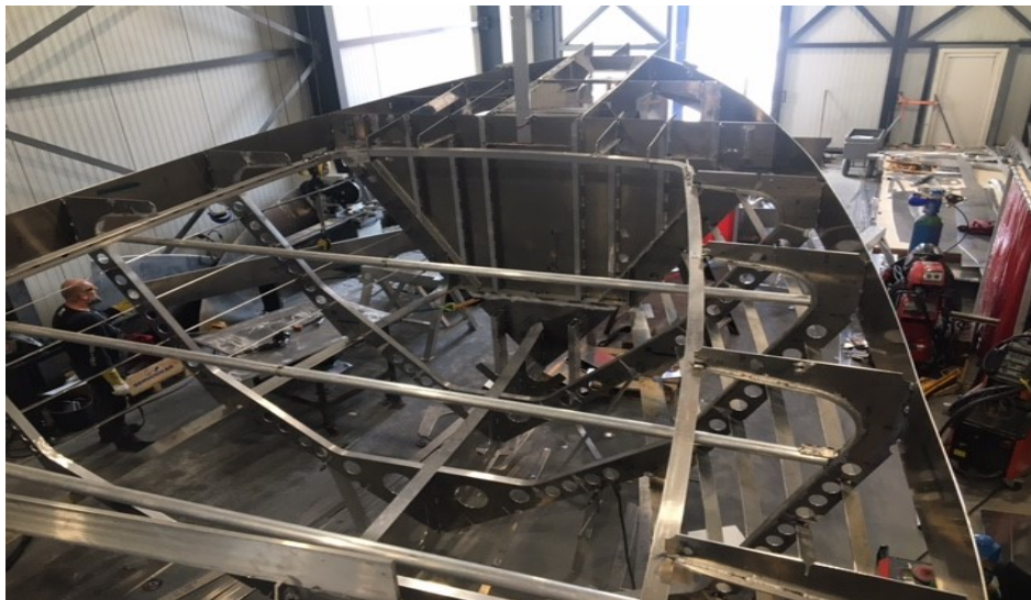
State of affairs in mid-August. Top: engine room with foundation at front left. Bottom: the bow and anchor hold begin to take shape. ©FH
