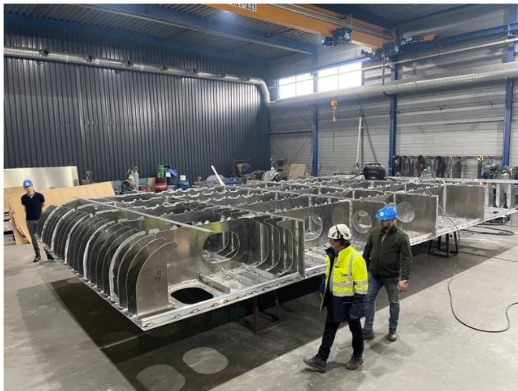
Construction of the first section of the RV Wim Wolff at N. Dijkstra in Harlingen in late October. ©FH
