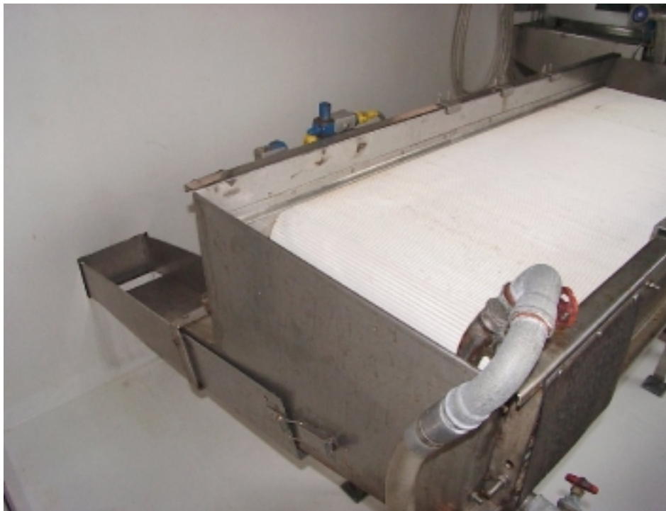
Inside view: seawater connection for flushing and cleaning
