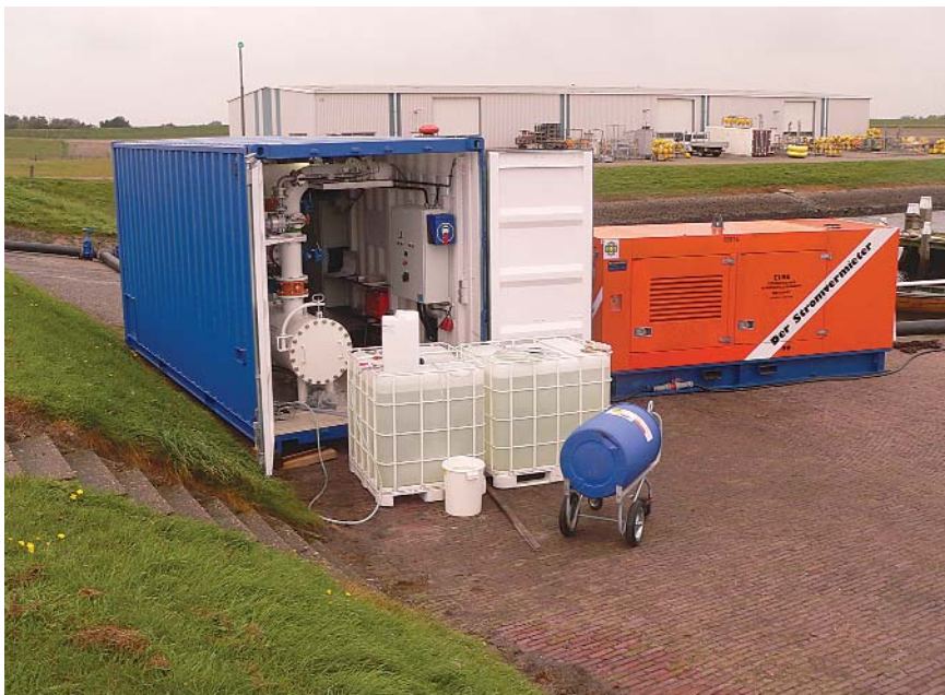
Fig. 2. The Ballast Water Treatment system temporarily installed at the NIOZ harbour.
