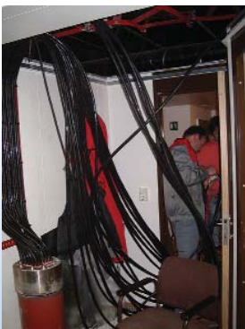
Almost 1.000 m of electrical cables had to be laid in the vessel
