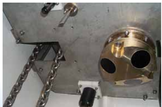
Current sensors at Texel ferry monitoring platform
